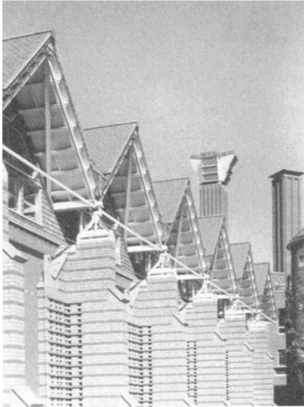
13.7 Mechanical laboratory showing buttress side wall vents with classroom exhaust stack and boiler flue behind.
